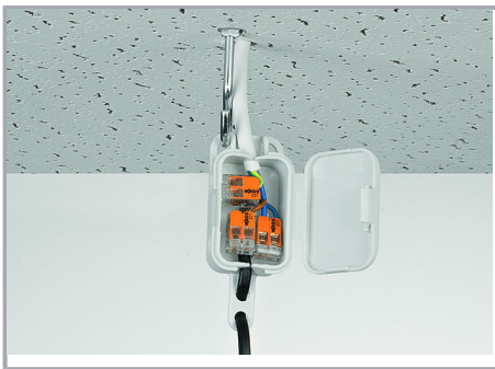
Pendant light connection in a suspended ceiling
