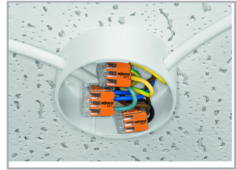
Lighting distribution in a ceiling canopy
